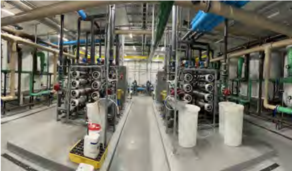
Commercial Water Treatment Plant after expansion
