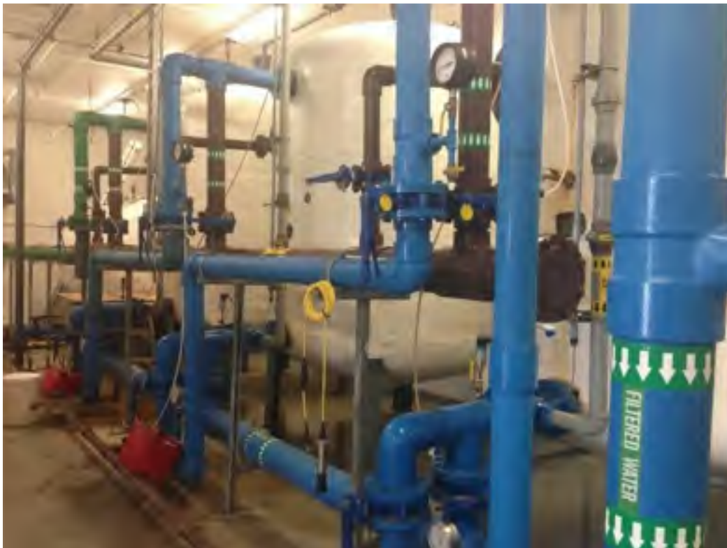
Commercial Water Treatment Plant prior to expansion
